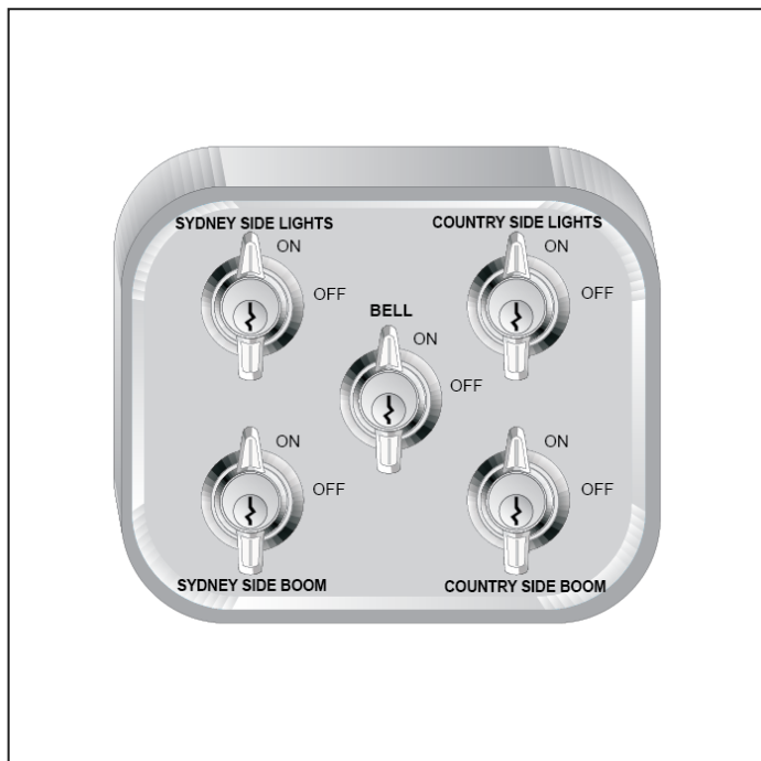
FIGURE 7: Emergency switch box with individual switches for lights, bell, and booms.
