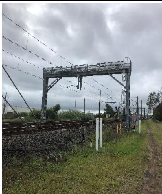
Image 5: Pantograph Condition Monitoring System (PCMS)
