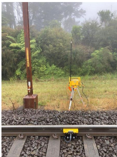
Image 1: Sensor and transmitter installation location
