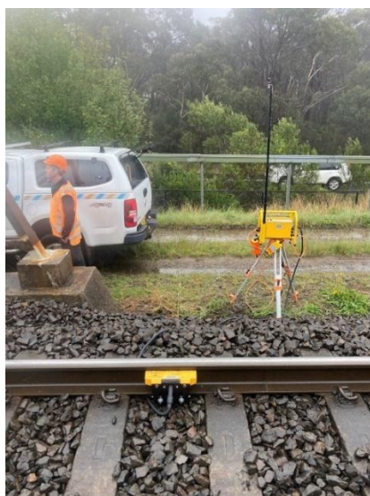
Image 1: Sensor and transmitter installation location
