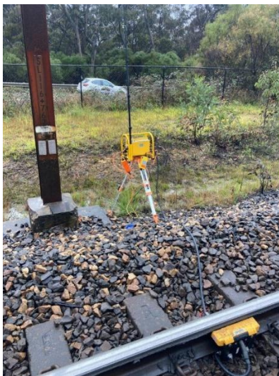
Image 1: Sensor and transmitter installation location
