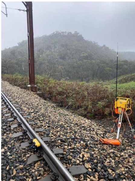
Image 1: Sensor and transmitter installation location
