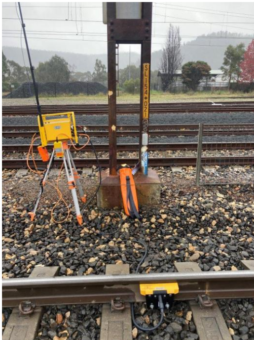
Image 1: Sensor and transmitter installation location
