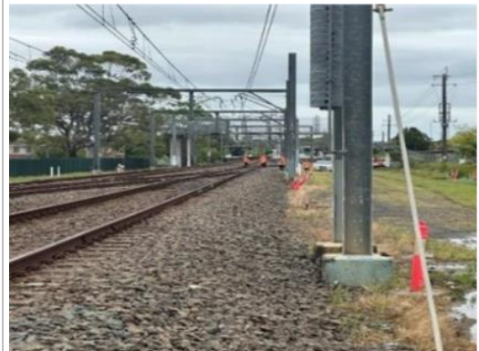
Image 2: View of worksite on the up towards East Hills station facing the Down direction.
