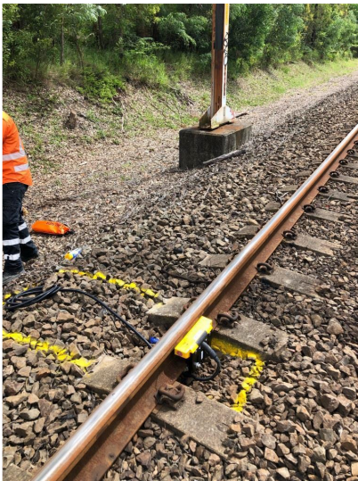
Image 1: Sensor and transmitter installation location
