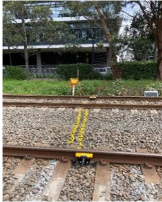
Image 1: Transmitter and sensor installation location
