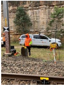
Image 1: Transmitter and sensor installation location
