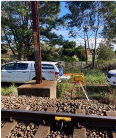
Image 1: Sensor and transmitter installation location
