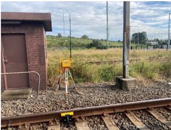
Image 1: Transmitter and sensor installation location
