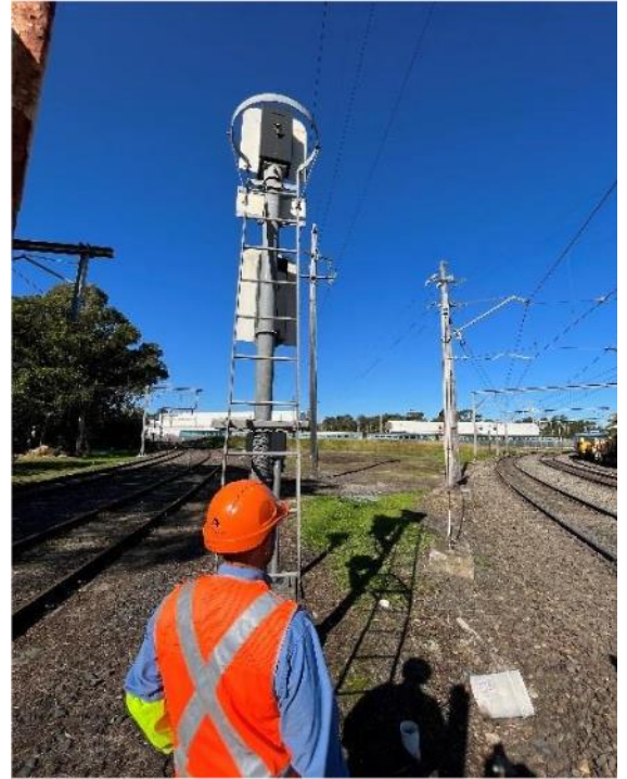
Image 2: Lookout position at SM 701 Signal facing both the North Forks and Goods lines
