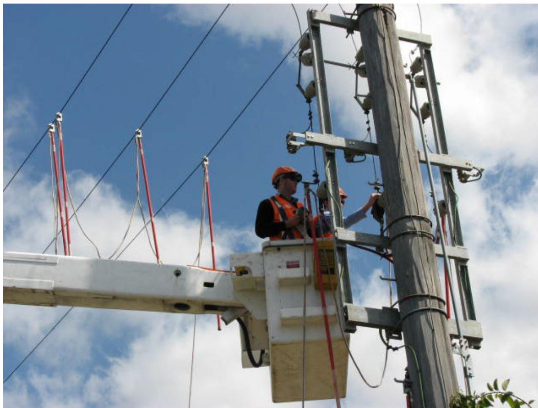
Figure 2 - Example of Installed Aerial Line Earthing Set
