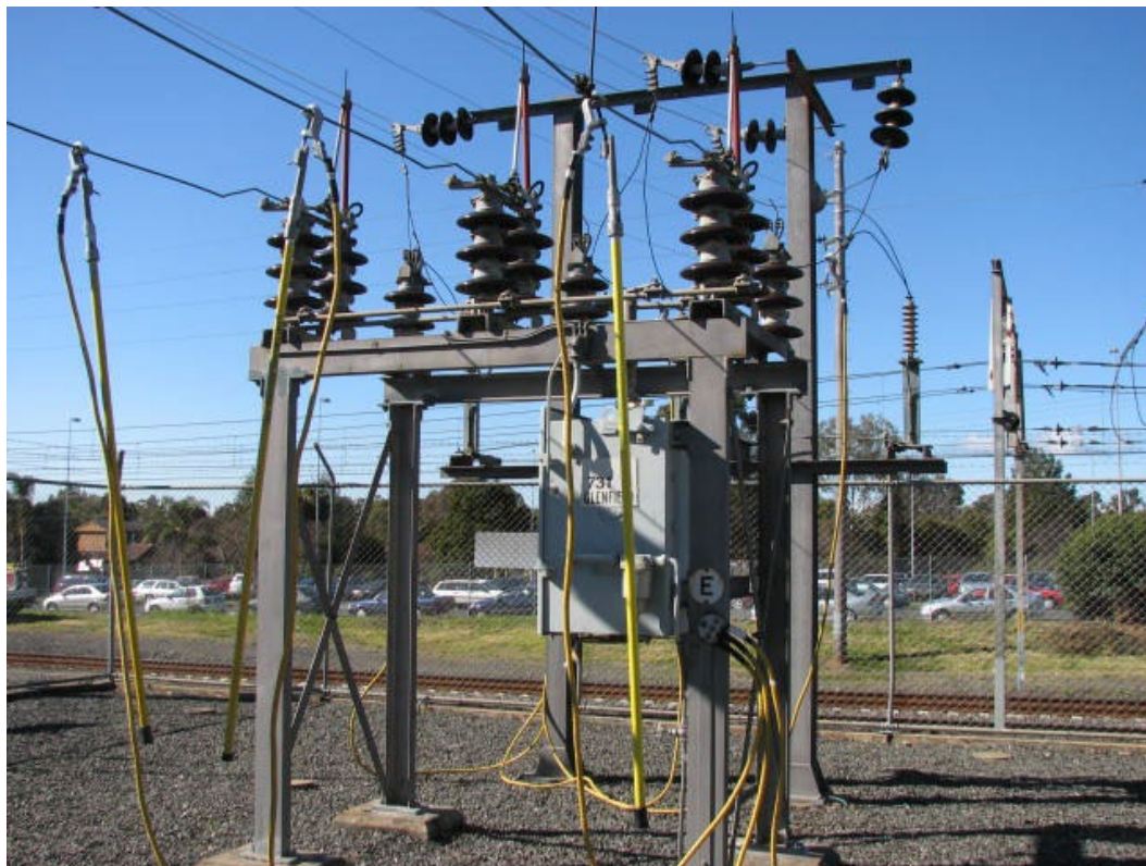
Figure 1 - Example of Installed Substation Earthing Set
