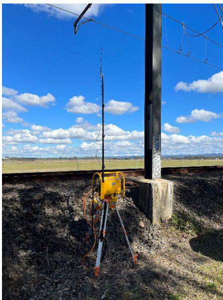
Image 1: View of Sensor 58.331 Richmond Main line
