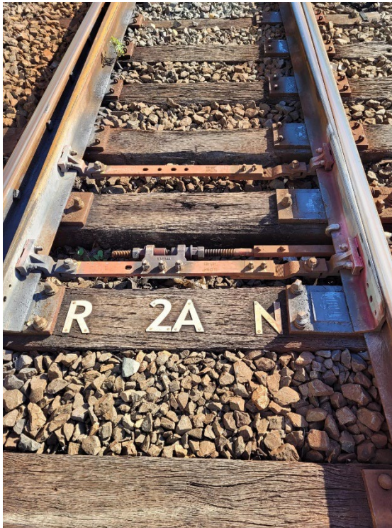
Image 3: Example of 2A points clipped and locked in the normal position to prevent rail traffic entry into the worksite.
