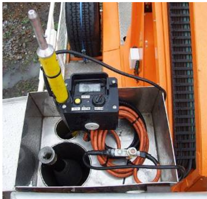
Negative Lug Attached to an Approved Rail Connection Bolt on an EWP
