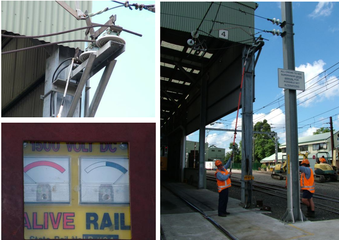
LR Tester Checking Continuity of Rail-Connecting Cables at 1500V Field Switch
