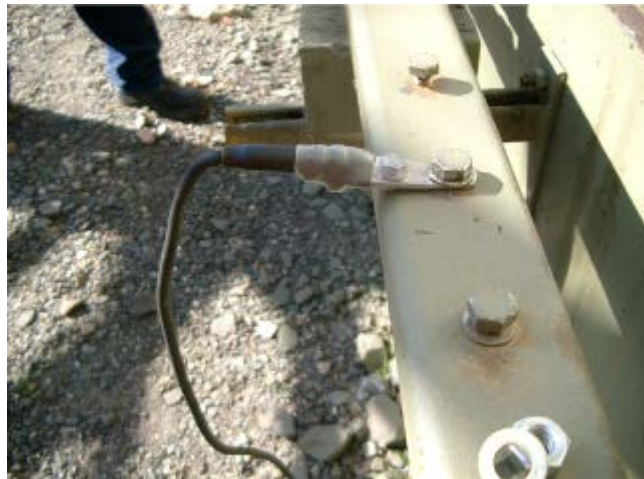
Negative Lug Attached to a Bolt on Test Rail
