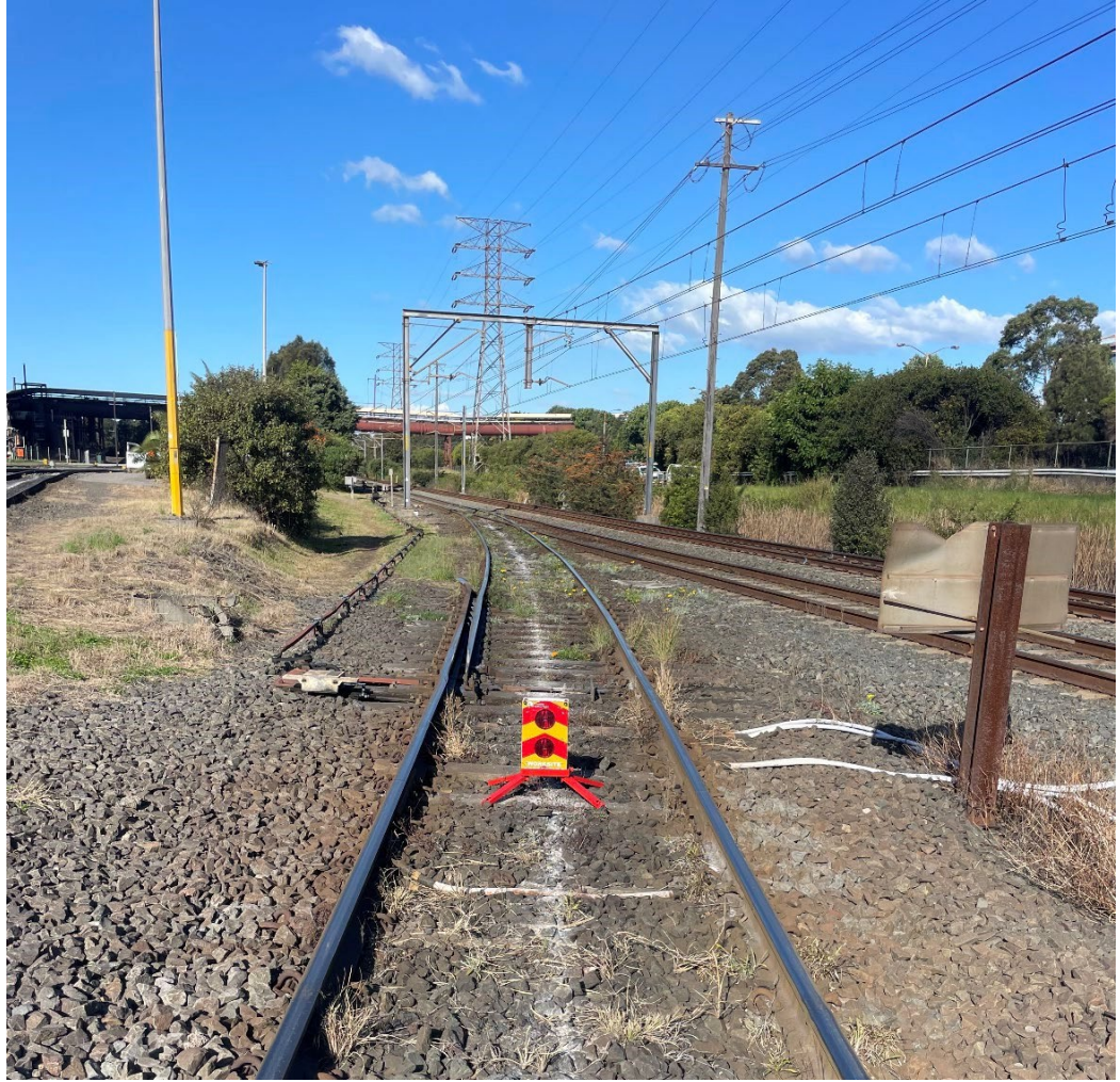
Image 3: Worksite Protection Marker placed clear of 531 Points (531 points clipped and locked by BlueScope Road Control)
