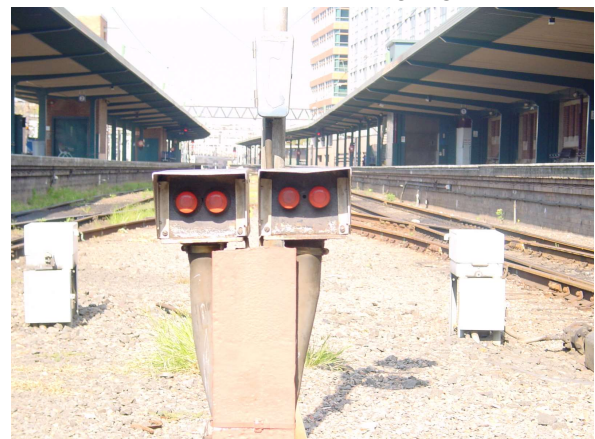
SHUNTERS PUSHBUTTON BETWEEN 1 AND 2 PLATFORMS
