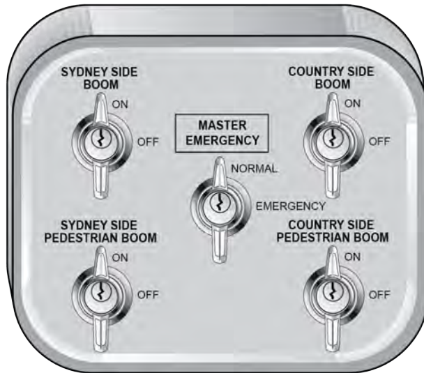
FIGURE 8: Emergency switch box with Master Emergency Switch and boom switches only. NOTE: Additional boom switches only provided if crossing is fitted with pedestrian booms
