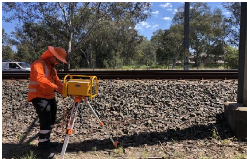
Image 2: Transmitter and sensor installation location
