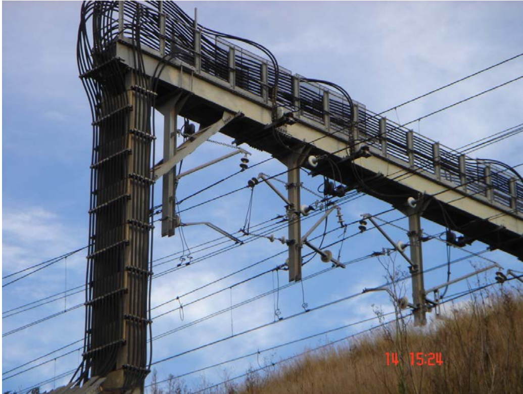
Figure 3 – An example of a feeding arrangement from the Substation to the Overhead Wiring
