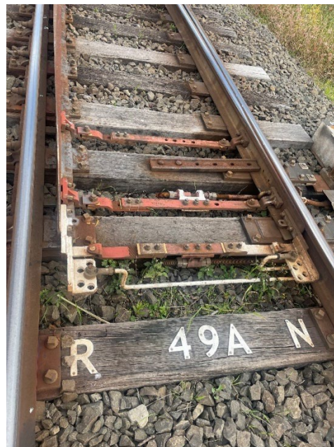
Image 8: Protection Officer must make sure that 49A points remain spiked this RNMWPP does not cover Wongawilli Colliery Siding
