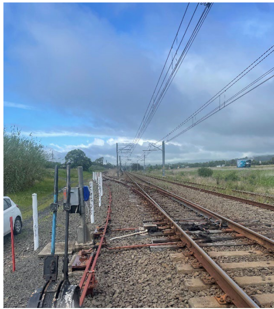
Image 5: Lookouts view from B Frame facing Kiama on the Kiama side of the Worksite
