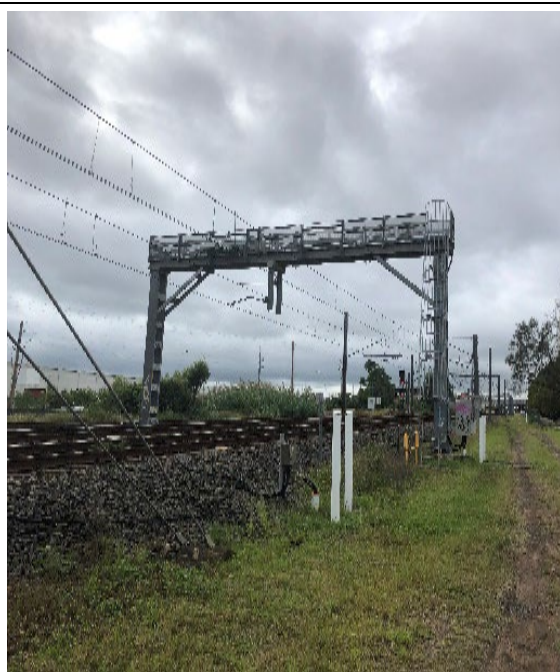
Image 5: Pantograph Condition Monitoring System (PCMS)
