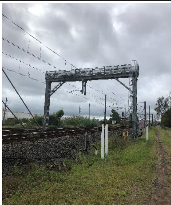
Image 5: Pantograph Condition Monitoring System (PCMS)
