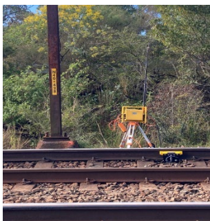
Image 1: Transmitter and sensor installation location
