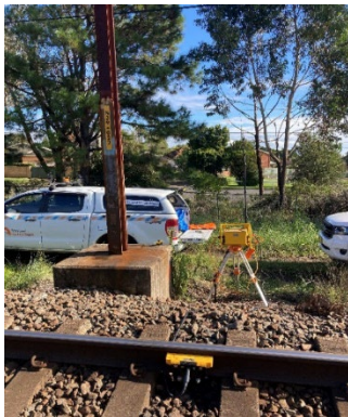
Image 1: Transmitter and sensor installation location
