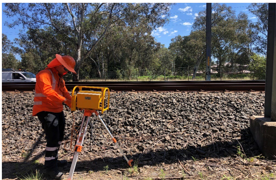
Image 2: Transmitter and sensor installation location
