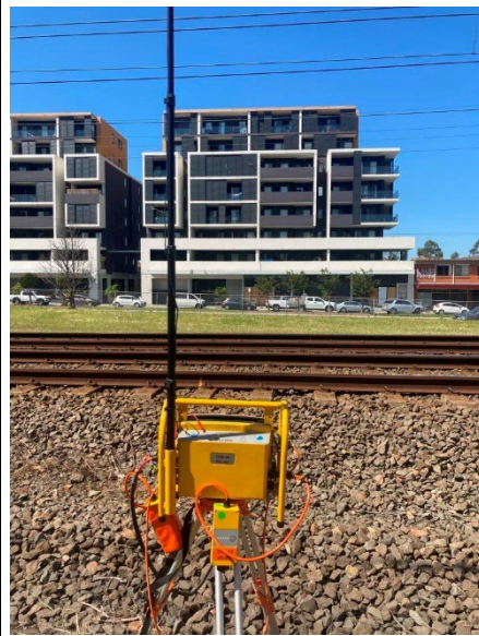
Image 2: Sensor installation location
