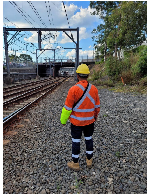
Image 8: Lookout in Up Cess for approaching rail traffic from the Up direction.
