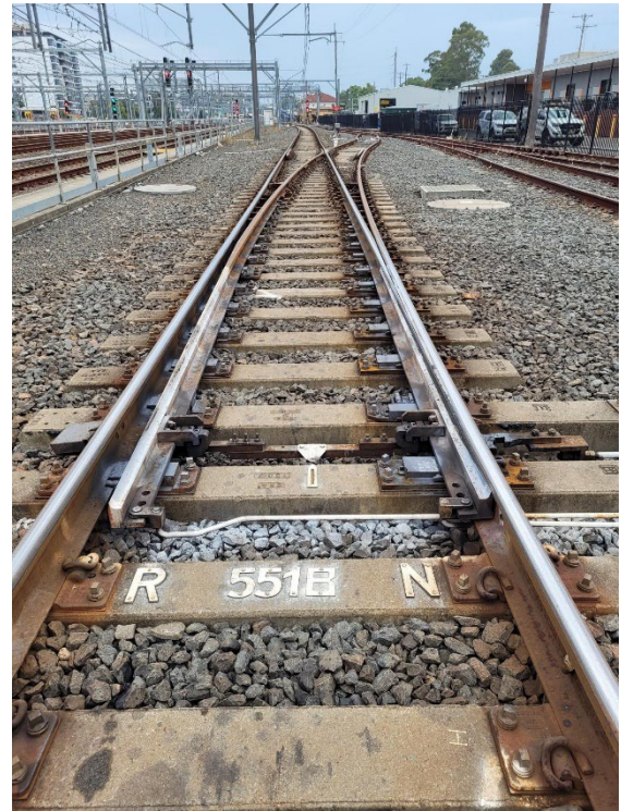
Image 6: (Live adjacent line): View of 551B points in the normal position from Down Relief leading into worksite. These points are to be clipped and locked in the normal position to prevent entry into the worksite.
