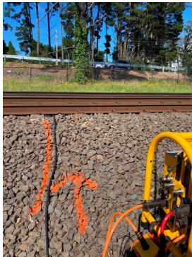
Image 1: Sensor and transmitter installation location
