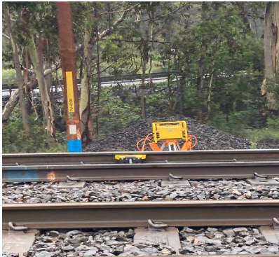
Image 1: Sensor and transmitter installation location
