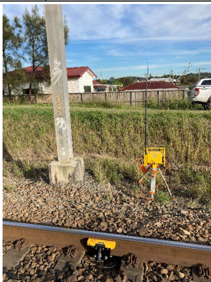
Image 1: Transmitter and sensor installation location
