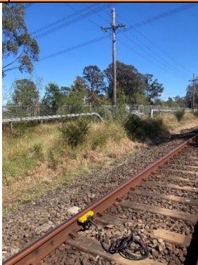
Image 1: Transmitter and sensor installation location
