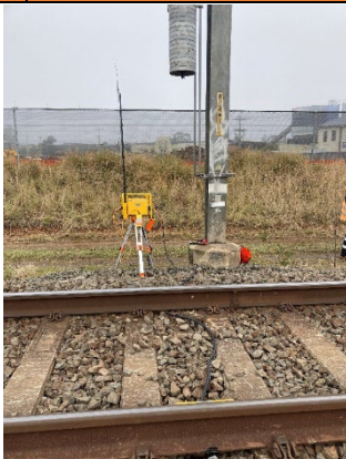
Image 1: Transmitter and sensor installation location
