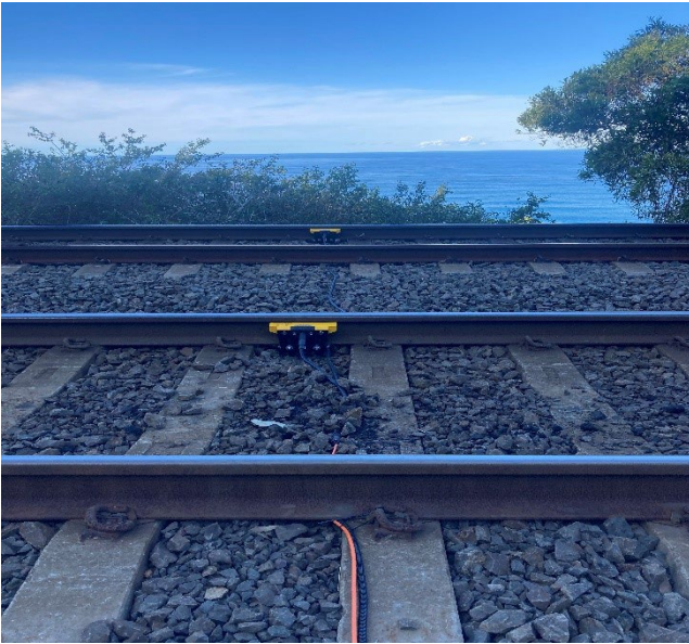
Image 1: Transmitter and sensor installation location
