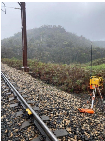
Image 1: Transmitter and sensor installation location
