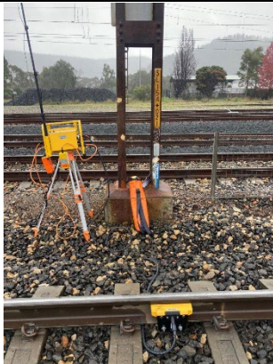
Image 1: Transmitter and sensor installation location
