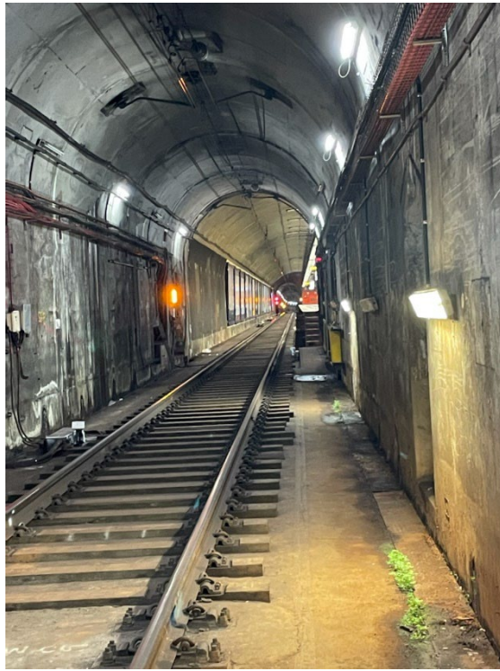
Image 1: Example of warning light at Bondi Junction and access by station platforms
