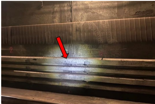
Asbestos containing troughing within the ESR.
