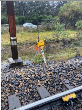
Image 1: Sensor and transmitter installation location
