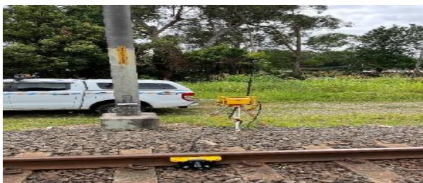
Image 1: Transmitter and sensor installation location
