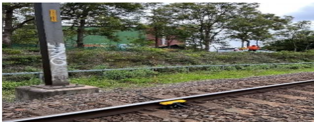
Image 1: Transmitter and sensor installation location
