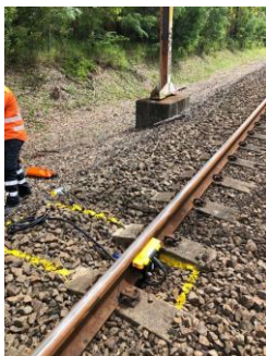
Image 1: Sensor installation location
