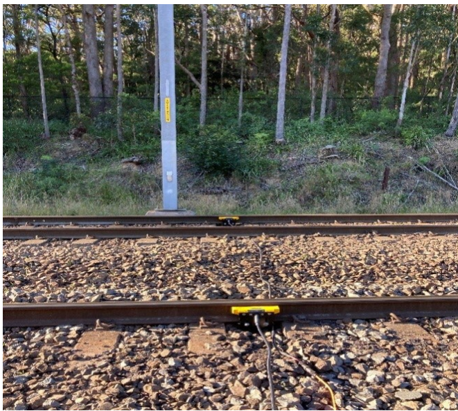
Image 1: Transmitter and sensor installation location
