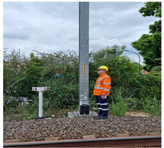
Image 4: Lookout position on the Down Bankstown line at 19.000 KM watching for rail traffic on the Down Bankstown line , for work on 363 points .
