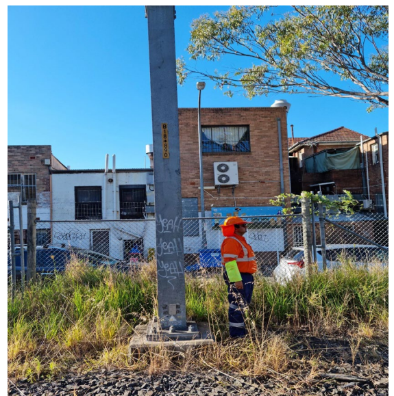
Image 2: Lookout position on the Down Bankstown line at 18.890 KM watching for rail traffic on Up Bankstown , for work on 361 points and 362 points .
