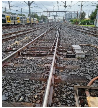
Image 9: Lookout view at 62A points . Watching rail traffic approach from the Country direction.
