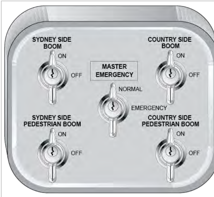
FIGURE 8: Emergency switch box with Master Emergency Switch and boom switches only. NOTE: Additional boom switches only provided if crossing is fitted with pedestrian booms.
