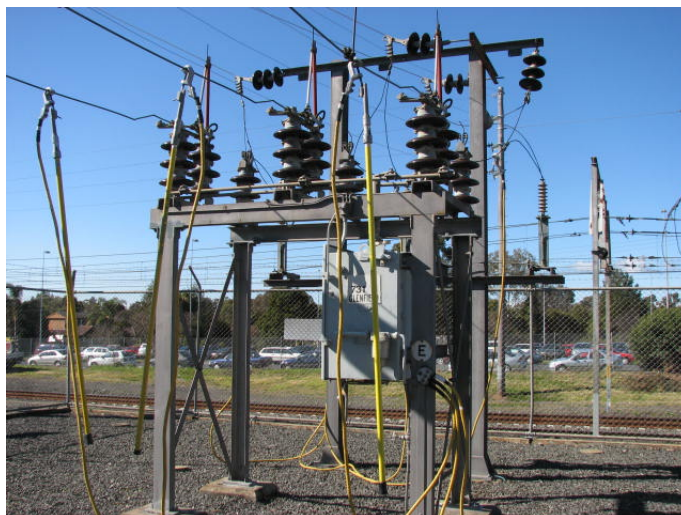
Figure 1 – Example of Installed Substation Earthing Set
