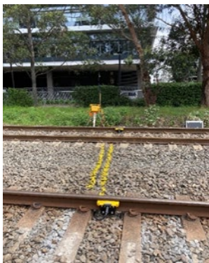
Image 1: Transmitter and sensor installation location
