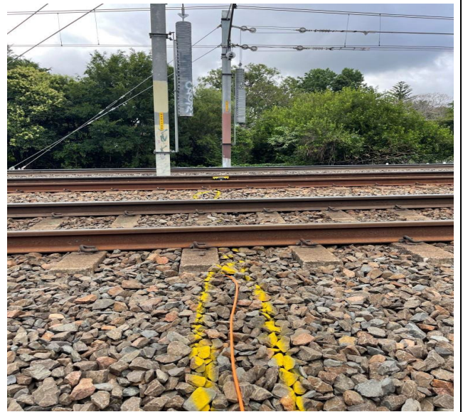
Image 2: Transmitter and sensor installation location.
