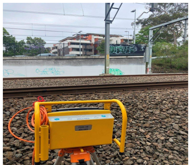
Image 2: Transmitter and sensor installation location.
