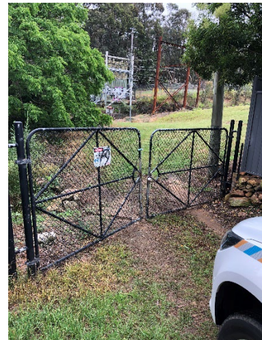
Image 5: Access gate W00 63.029 D to 38.9 Signal
