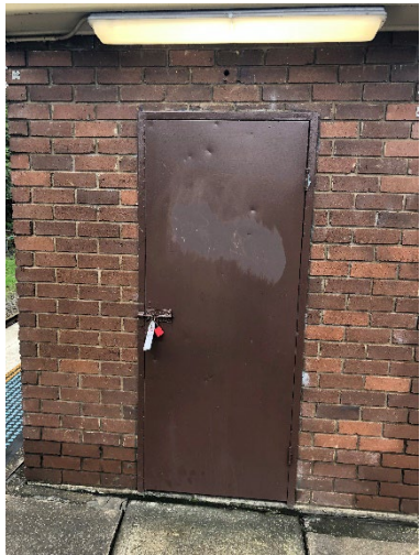
Image 1: Danger tag and dedicated padlock on Glenbrook control panel door.
