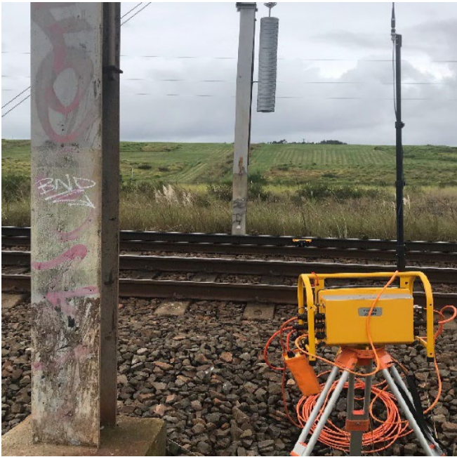
Image 1: Transmitter and sensor installation location
