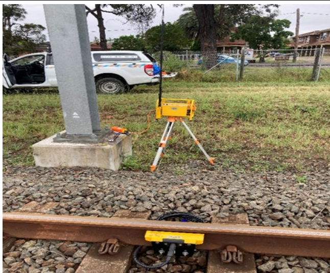
Image 1: Sensor and transmitter installation location
